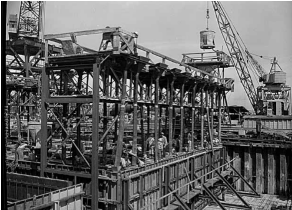
Evergreen Point Bridge pontoons under construction, Seattle, May 1961. Courtesy Museum of History & Industry.
